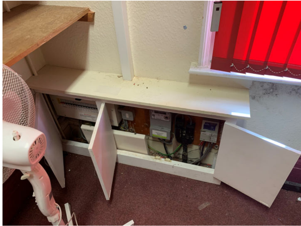
The Lodge – Incoming supply from DNO
