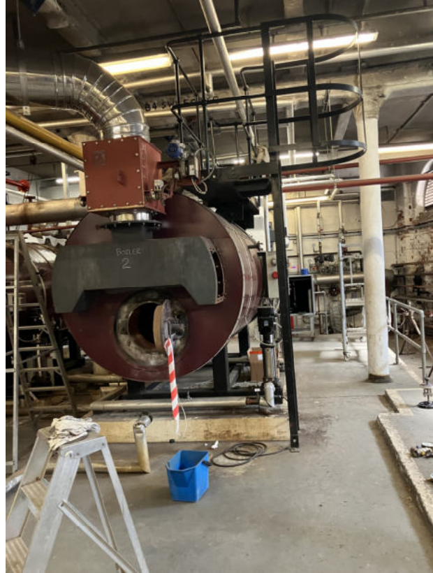
South Block Boiler House – Large Boiler
