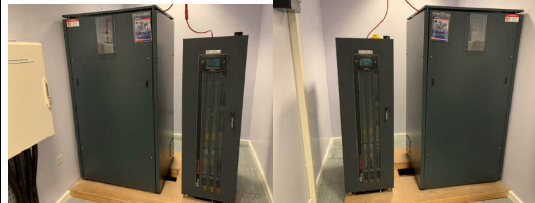
South Block UPS
