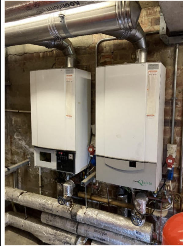
South Block - Boilers
